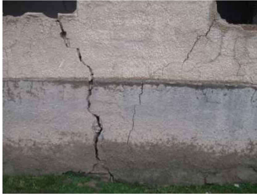
Figure 2. A crack formed as a result of uneven subsidence of the soil of the building. In the case of small and relatively low-risk cracks in the walls of the building, such as landslides in the upper layer of plaster, it is possible to eliminate existing damage by re-plastering and painting.
